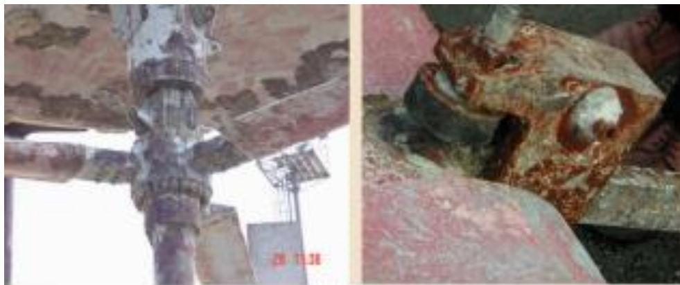
Figure 11 Corrosion profile of HK turbine
